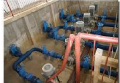
Impressive pumping station at Manyonyo. Some minor issues with debris / silt entering the foot valves
