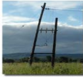
Temporary setback: ZESCO removed transformers recently at Sinazongwe and Nzenga
