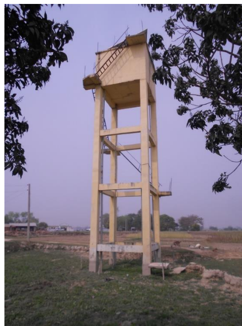
Figure 3 Unused OHT scheme in Silautiya, Rupandehi
